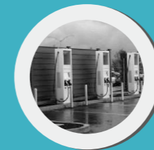
充电桩 Charging Pile
